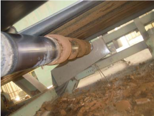
Conch Cement had excessive spillage on the return belt on the conveyors transferring limestone and clay.
