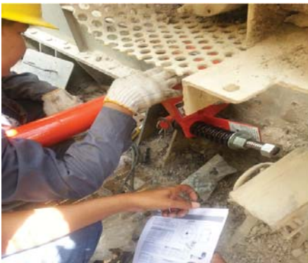
Martin Engineering technicians install the Martin® QC1™ HD cleaner on the underside of the head pulley.
