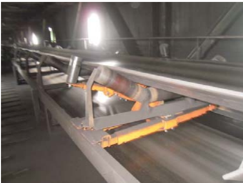
The Martin® Trackers™ have corrected the alignment issues and have increase plant efficiency.
