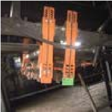
Martin Engineering installed Martin® upper Tracker™ & Martin® lower Tracker™ to correct the problem.
