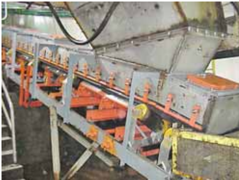
Following the project, transfer points at the Alcoa's Warrick Power Plant featured new chute work, improved support and skirting systems.
