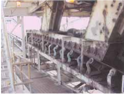
This is a typical transfer point at Alcoa's Warrick Power Plant before the MartinPLUS® Services reconstruction project.
