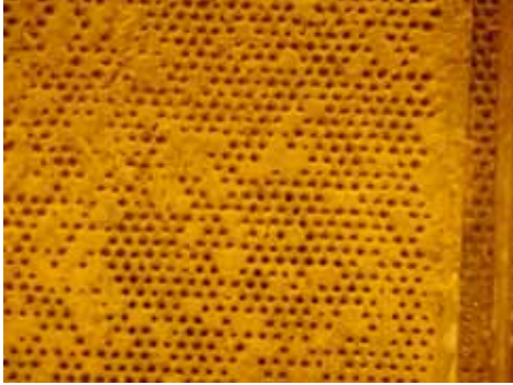
Screen from chips dryer, showing sawdust plugging.
