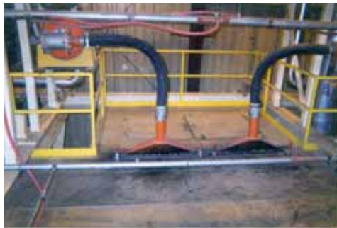
To allow the Martin® Air Cannons to clean two of the screens, special discharge nozzles were installed.
