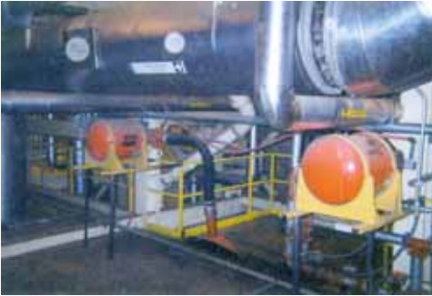
Martin® Air Cannons were installed so their discharge would remove the buildup from the dryer screens.
